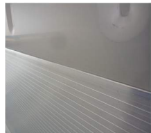
The connection between the lining and the scufflining is without visible sealant.
