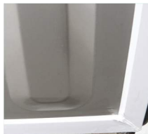
No visible sealant inside the doors
